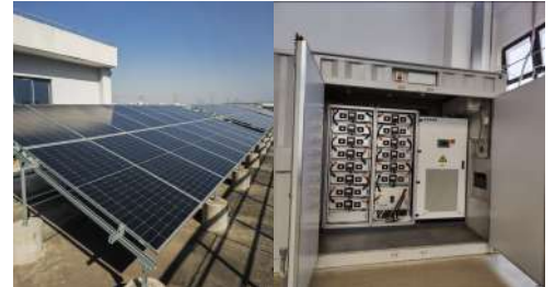
New Energy EPC Project
